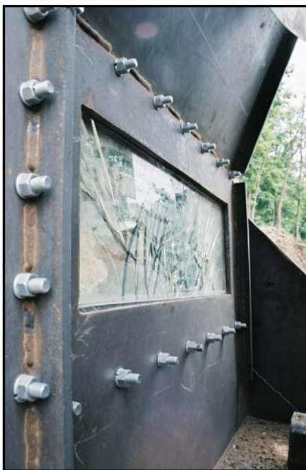
Figure 19. Interior of Glass After Second Blast
