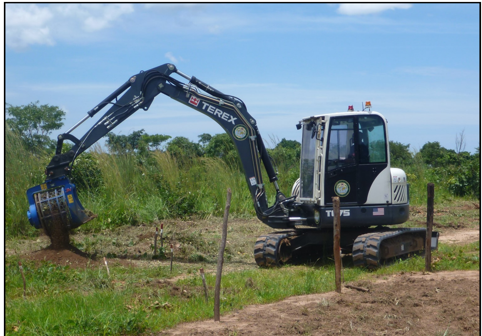
REX with its mine sifting bucket attachment in Angola during initial operator training with MAG deminers
